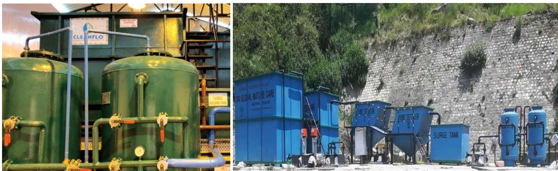
Figure 9 Sewage Treatment Facility at Jhakri Village
