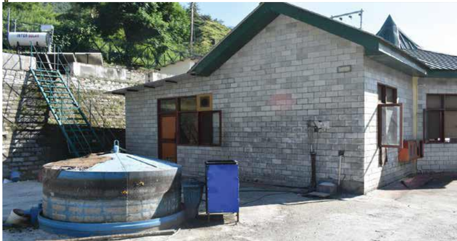
Figure 11 Biogas Plant for Office Canteen, Jhakri
